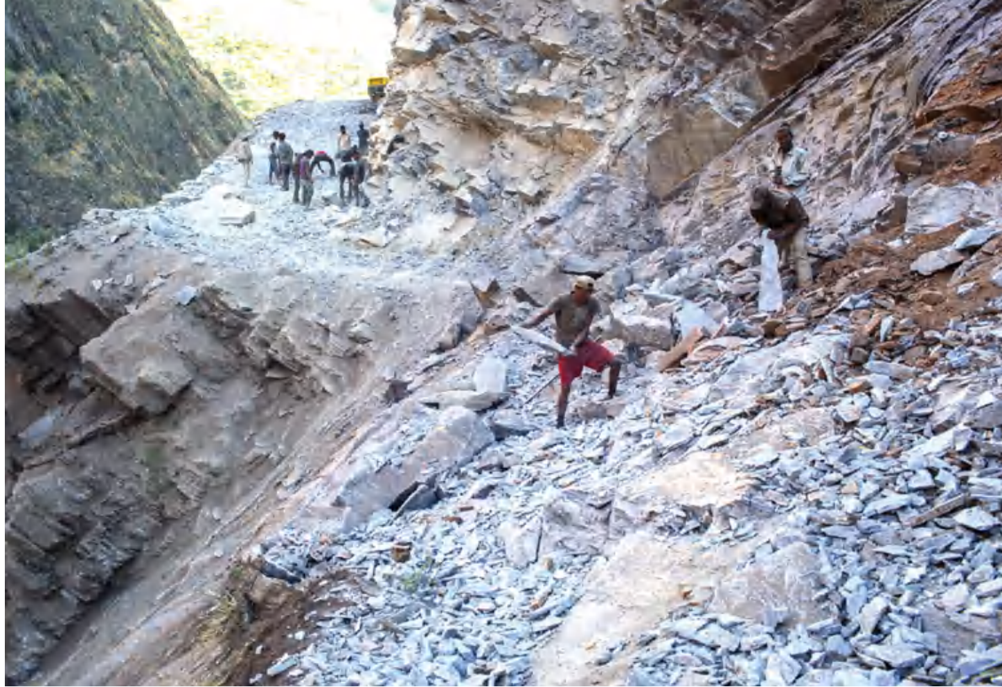
Road construction alignment along major river channels adds chronic sediment to streams reducing aquatic habitat and unstable terrain threatens the longevity of the road system.
