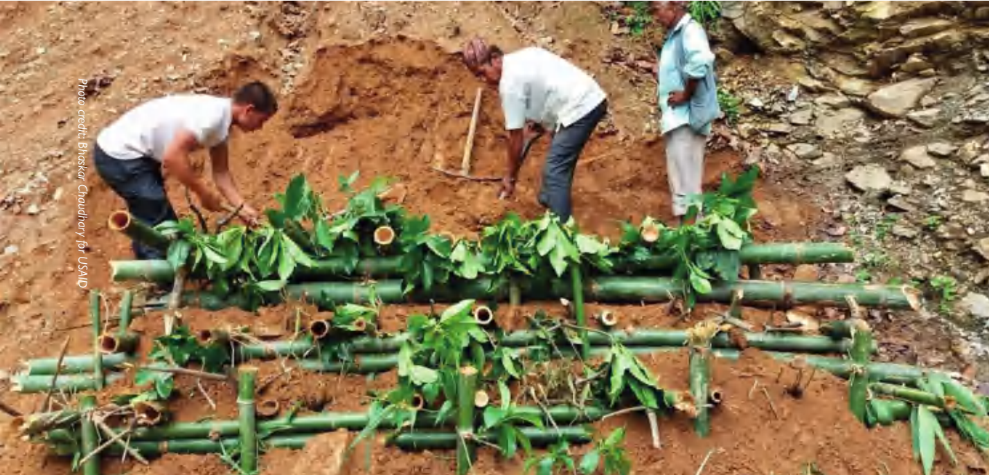
Participants learn how to build bamboo crib walls on road side slopes to increase soil stability and combat landslides in a bio-engineering training organized by Paani
